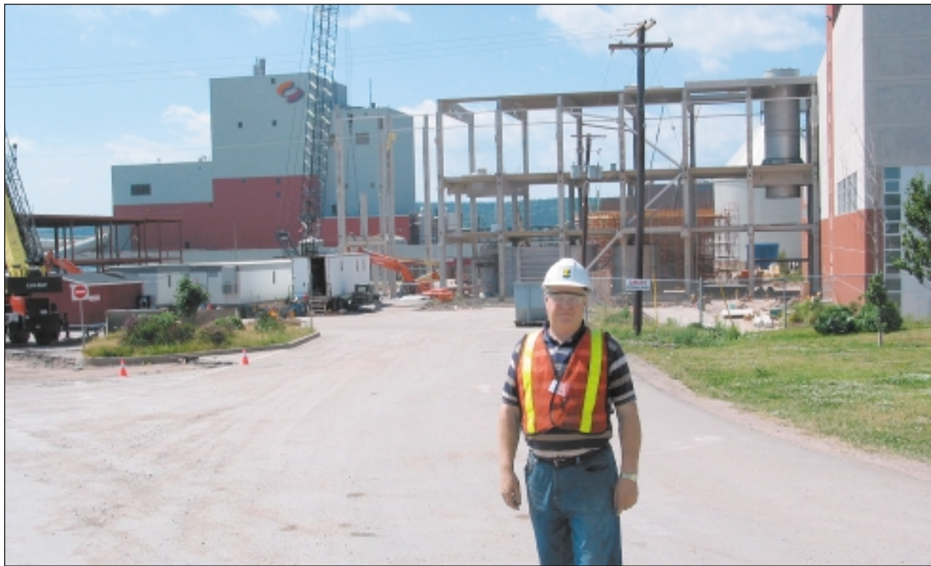
The StoraEnso pulp and paper mill, Port Hawkesbury, N.S. is undergoing a multi-million dollar expansion to modernize and increase its production capacity. Ted van Zutphen, co-owner of J&T van Zutphen Construction Inc., the general contractor for the largest phase of this project, took time to give a brief site tour last July. The firm's ready mix company, Ideal Concrete Ltd., will provide over 7,700 m 3 of concrete for this job.
