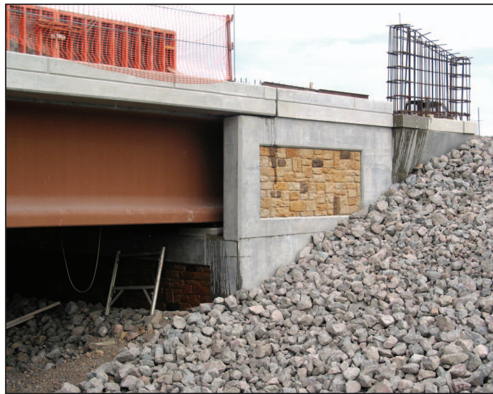
The new Petitcodiac River Bridge between Moncton and Riverview, New Brunswick was opened to traffic on November 19, 2005. The project featured several innovative concrete construction techniques, including the use of self-consolidating concrete (SCC), form liners and acid-stain colour to provide a durable, detailed, coloured stone pattern for the barrier walls.
