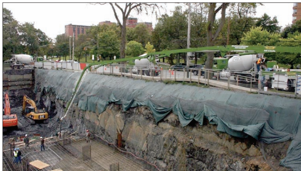
Ocean Contractors will use close to 15,000 cubic yards of concrete for the Trillium project, an 84-unit condo on South Park Street in Halifax, Nova Scotia.
