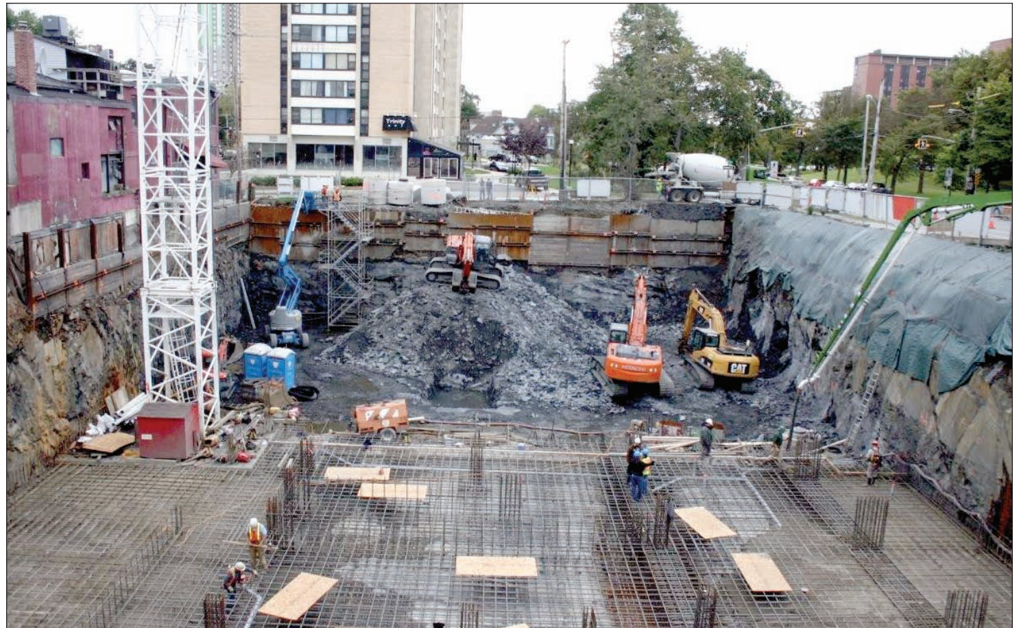
The Trillium project on South Park Street is one of the largest residential building projects in downtown Halifax's recent history. See the story on page 4.
