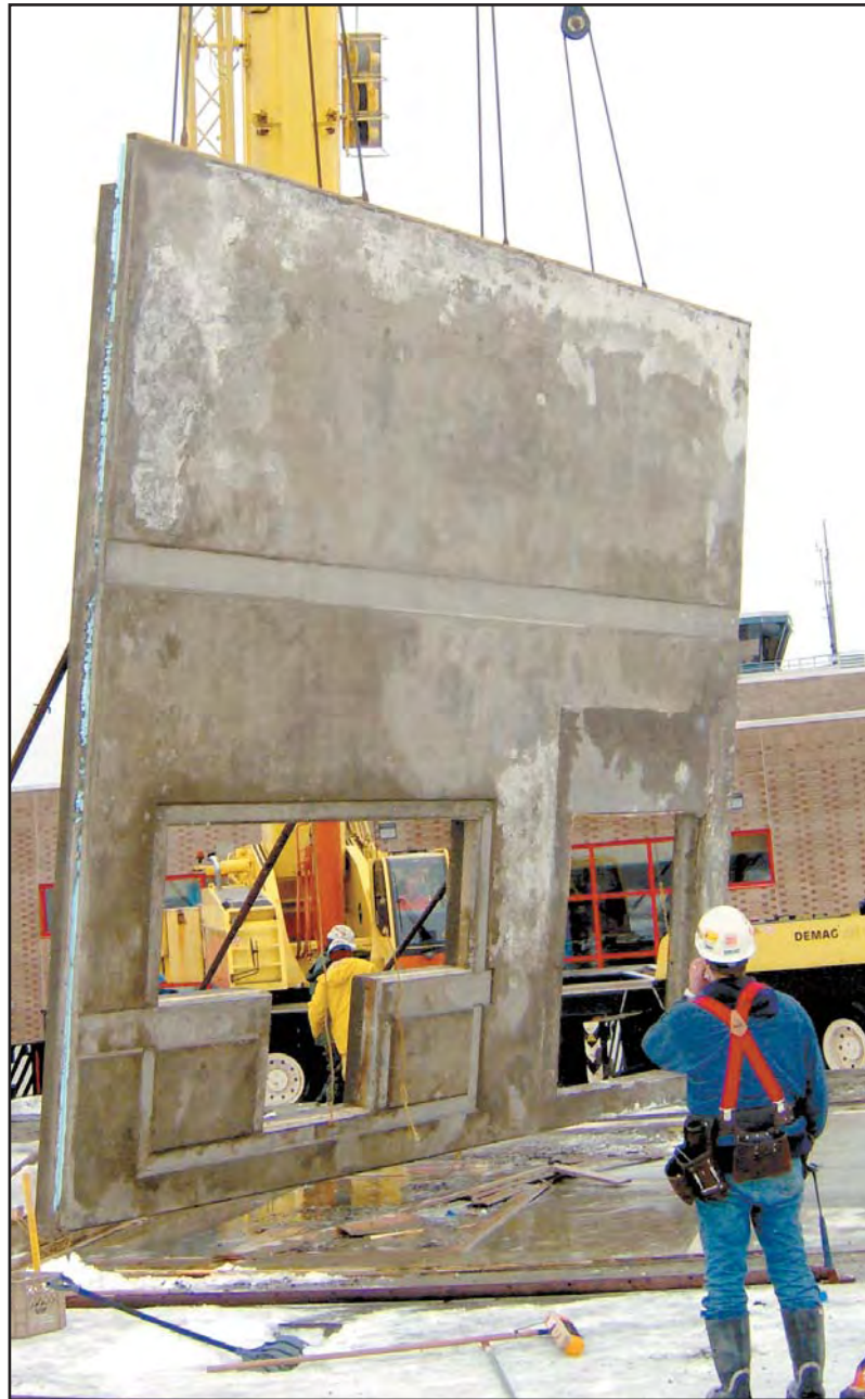
The extension to the Fredericton Airport, the first government/institutional tilt-up project in New Brunswick, was completed last winter (design consultant: ADI Limited; general contractor: Rideau Construction Inc.). David Beattie, ADI Limited, says they found the method to be cost effective, resulting in a durable building that's easier to heat and maintain.
