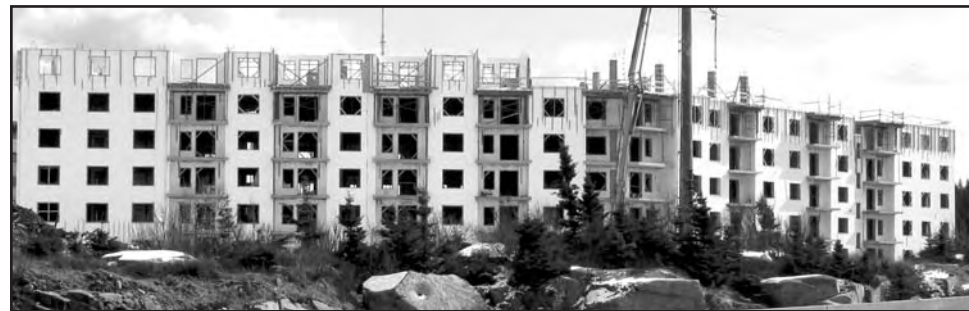
Sackville Concrete supplied the concrete for a six-storey ICF condo in Clayton Park, near the Bicentennial Highway, for property developers Steve and Peter Gianoulis. The project was built through the winter months. Factors for using concrete: greater heating efficiency with heat savings up to 40 percent; elimination of highway traffic noise; concrete stays warm during steady set in freezing temperatures; winter heat during construction was minimized.
