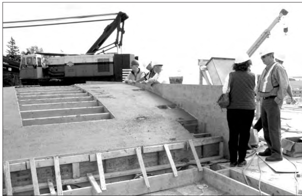
The APRMCA and CAC Tilt-up Concrete Symposium included a tour of nine tilt-up sites in the Halifax area to increase awareness of the advantages of tilt-up technology.
