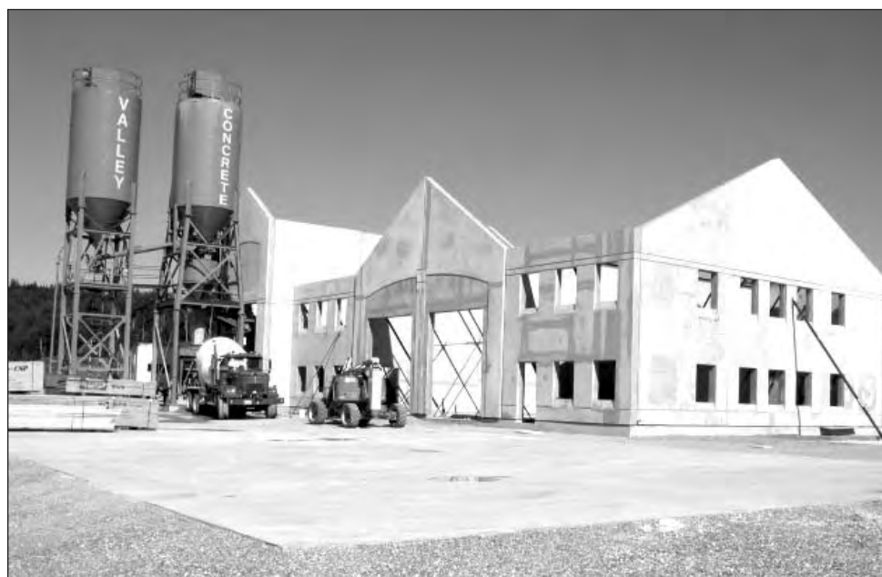
Fundy Contractors Ltd. of St George, N.B. put up a new plant called Valley Concrete Inc. in Quispamsis, N.B. in early summer. It commissioned B.D. Stevens Ltd. of Dartmouth, N.S. to build a tilt-up office and shop.
